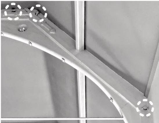
Guide wheels for operating the ventilation cowl.
